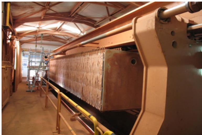
Filter bertekanan di Pengilangan Gardanne, France
